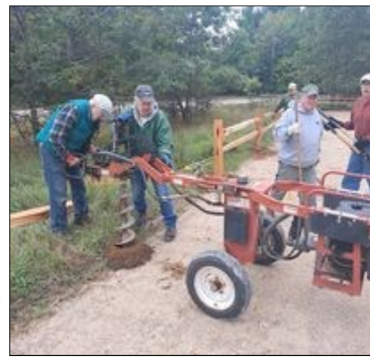
Volunteers drilled post holes in the final stages of creating a new parking lot at the Preserve.
